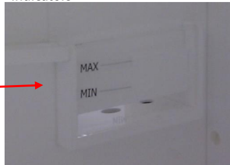
Figure 38: Water tank internal level indicators
